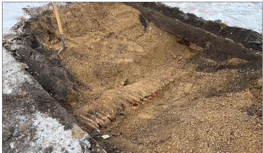
City officials were unaware of the condition of an existing irrigation line the sewer line crossed under. Due to its deteriorated condition, the irrigation line had to be replaced at every location that it was exposed.
