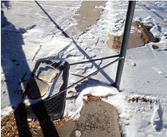
Figure 19 Observation shows stanchion supporting a pole that obstructs the clear width of the sidewalk.
