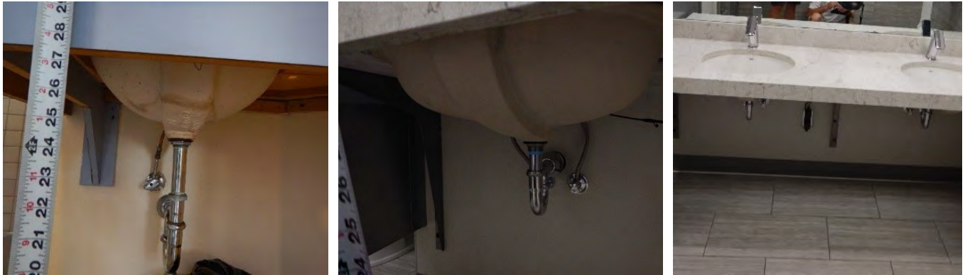
Figure 2.4.1.1(f) Typical Observation: Water supply and drain pipes are not insulated under lavatories: [ADA Standards 606.5. ]
