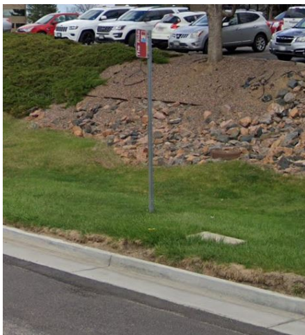
Figure 29 Bus stop sign posted at location without pad or connection to an accessible route.
