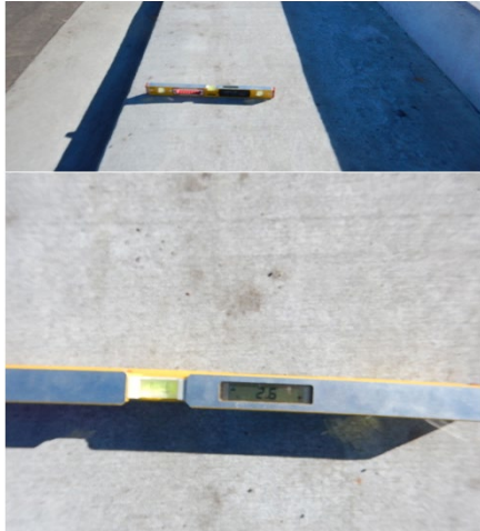
Figure 15 Measurement shows the cross slope of this sidewalk is 2.6%.
