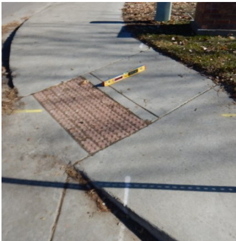
Figure 4 Diagonal curb ramp has no turning space.
