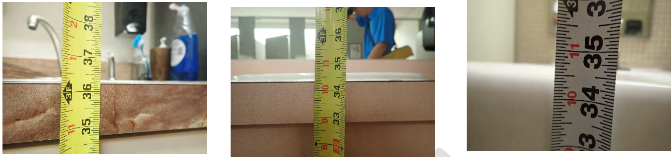
Figure 2.4.1.2(b) Typical Observation: Sink tops are too high: [ADA Standards 606.3. ]
