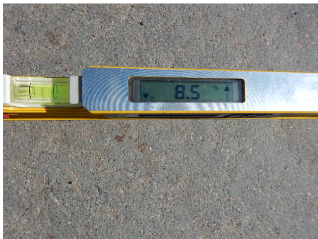
Figure 27 Measurement shows cross slope of sidewalk, at driveway, is 8.5%.
