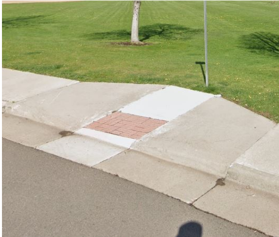
Figure 10 No turning space is provided at the top of this curb ramp.
