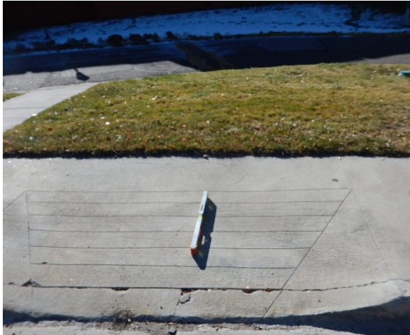
Figure 8 Detectable warnings are missing from this curb ramp.
