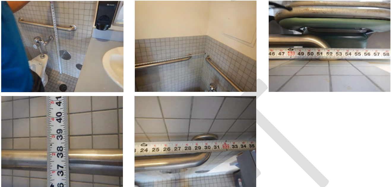
Figure 2.4.1.1(e) Typical Observation: improperly mounted grab bars in restrooms: [ADA Standards 604.5 and 609.4 .]
