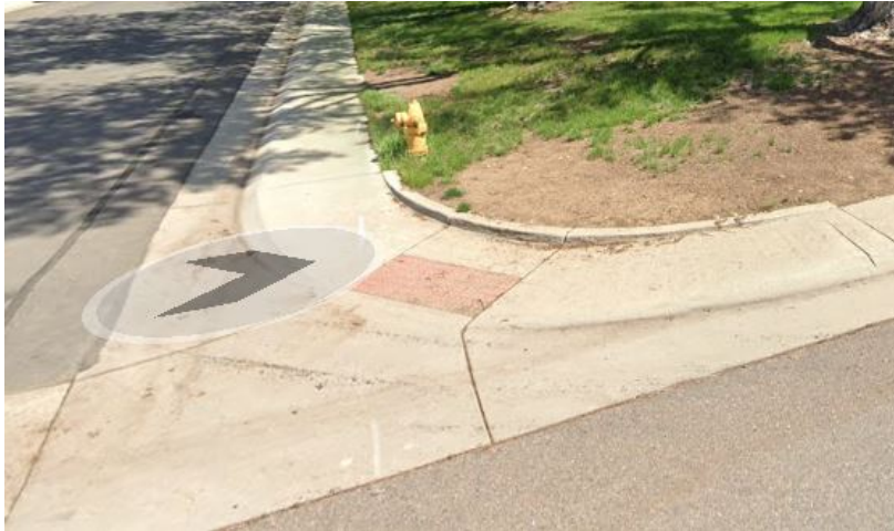
Figure 13 Turning space on this parallel curb ramp is too narrow.
