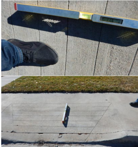
Figure 2 Measurement shows the running slope of this curb ramp is 11.5%.
