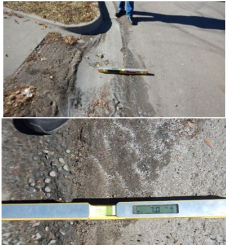
Figure 3 Measurement shows the counter slope of this curb ramp is 7.0%.
