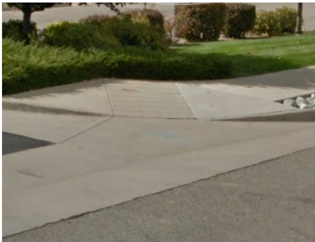
Figure 12 No turning space is provided at the top of this curb ramp.
