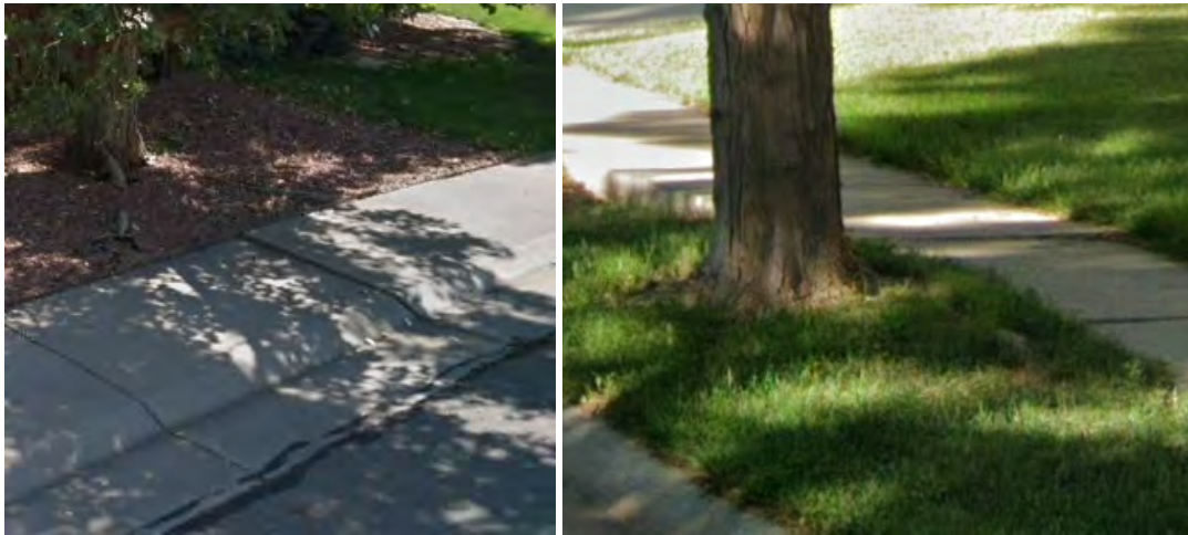
Figure 2.6.1.2(b) Typical Observation: Complex vertical discontinuity greater than 1.5 inches with cross slope steeper than 2.0 percent (1:50). [ PROWAG R3027.2. ]
