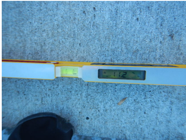
Figure 25 Measurement shows the running slope of the sidewalk, at driveway, is 11.2%.
