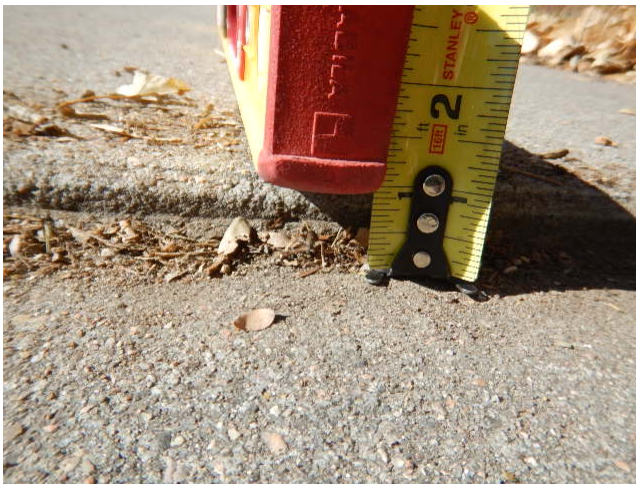
Figure 16 Measurement shows a vertical discontinuity greater than 1/2 inch.
