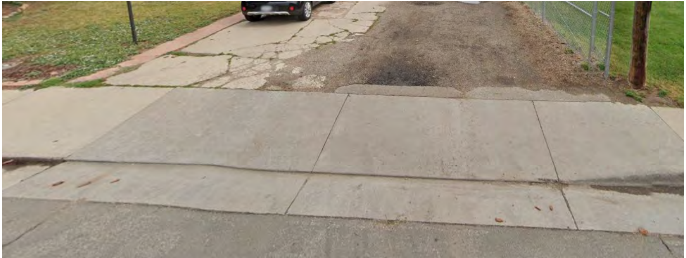
Figure 2.6.1.3(i) Typical Observation: Driveways at attached sidewalks create sidewalk running slopes steeper than 8.3 percent (1:12) and cross slopes steeper than 2.0 percent (1:50). [ PROWAG R302.5.1 and R302.6. ]
