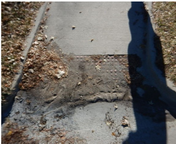
Figure 7 Detectable warnings are buried.
