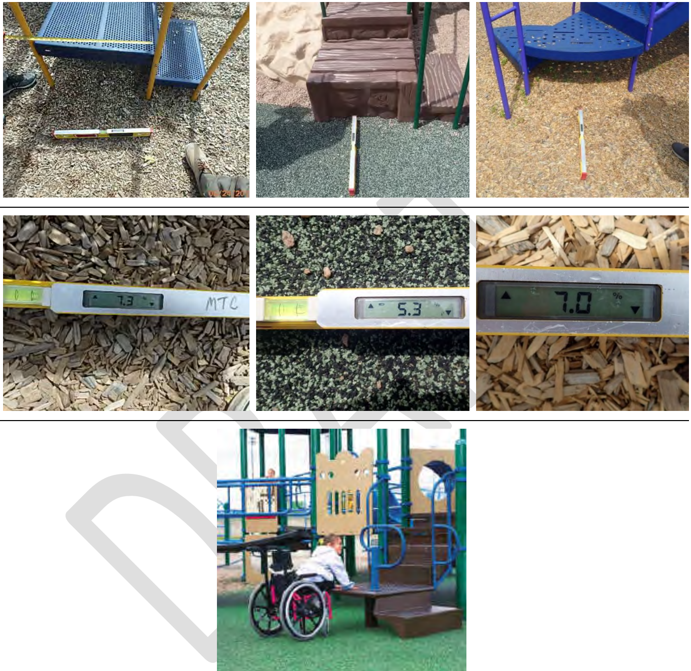
Figure 2.5.1.3(b) Typical Observation: Maximum slope of the transfer space at play area transfer platform is 9.1 percent. [ADA Standards 1008.3.1.3 and 305.2 ]
