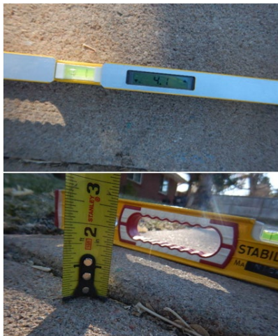
Figure 17 Measurement shows a vertical discontinuity greater than 1/2 inch where the cross slope is 4.1%.
