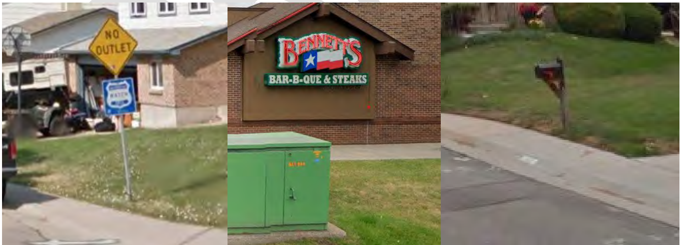
Figure 2.6.1.2(c) Typical Observation: Built features (such as signs and mailboxes) between 27 and 80 inches above a sidewalk, protruding more than 4 inches create a hazardous barrier for pedestrians who are blind or have low-vision. [ PROWAG R402.2. ]
