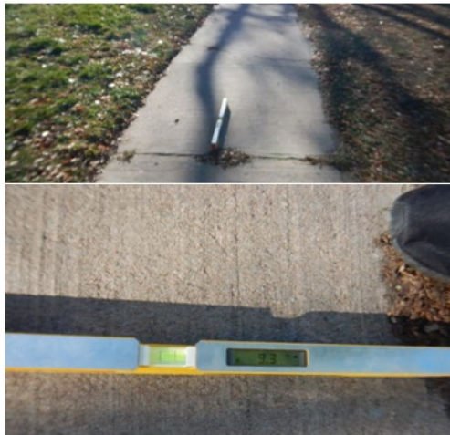
Figure 14 Measurement shows the running slope of this sidewalk is 9.3%.
