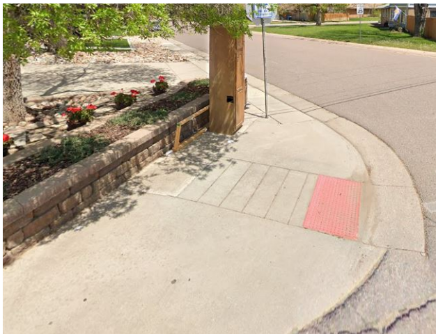
Figure 9 Turning space at the top of this curb ramp is too narrow.
