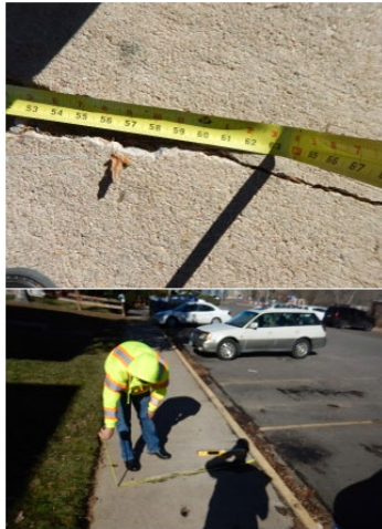
Figure 18 Measurement shows a horizontal opening greater than 1/2 inch across the width of the sidewalk.
